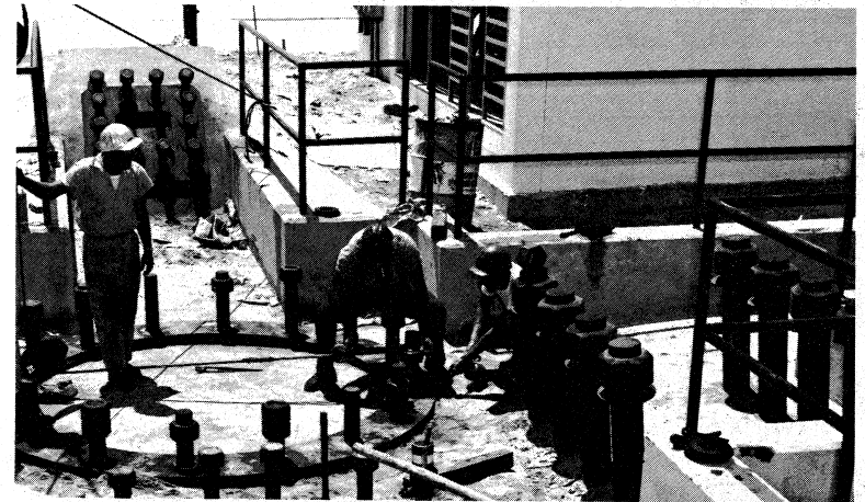
Anchor bolts mounted in 14-foot-thick concrete mat now hold support pedestals for Mobile Service Structure in its park position.
