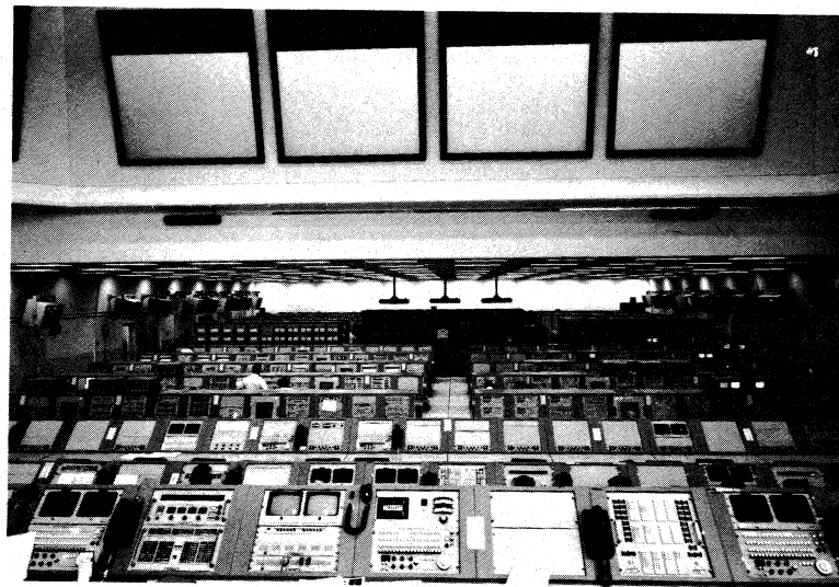
Interior of Firing Room 1, Launch Control Center, during installation of equipment consoles. TV monitors line walls on either side, with rearview, data projection screens above.
