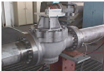
Valve water flow test
